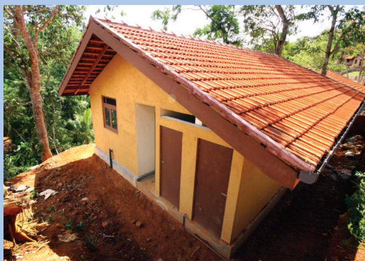
A house nears completion at Kongalahena. It is one of more than 22,000 houses completed to date in Sri Lanka with Red Cross Red Crescent support. A further 9,000 are under construction.
