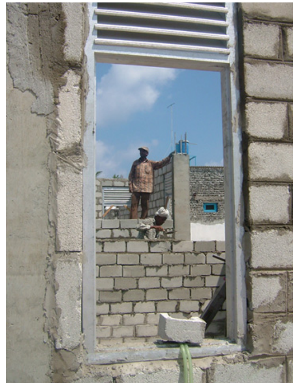
As the construction of permanent houses continues in the Maldives, the first completed homes have been handed over to tsunami survivors.
