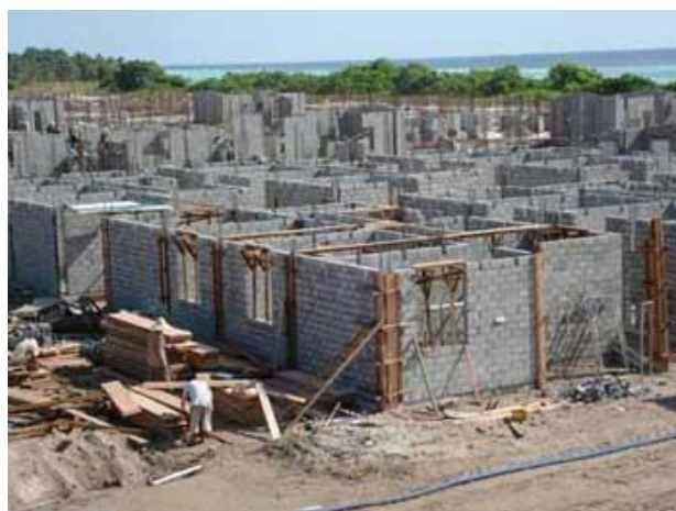
Houses going up on the 600-house scheme on Dhuvaafaru Island, The Maldives
