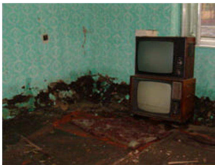
Aftermath: While some houses are still standing, the damages they suffered are irreparable and it is expected that they will collapse within a short time
