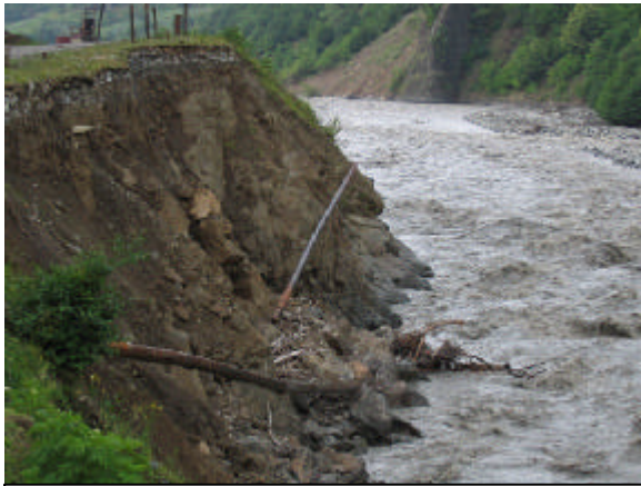
Destroyed water supply system in Oni region
