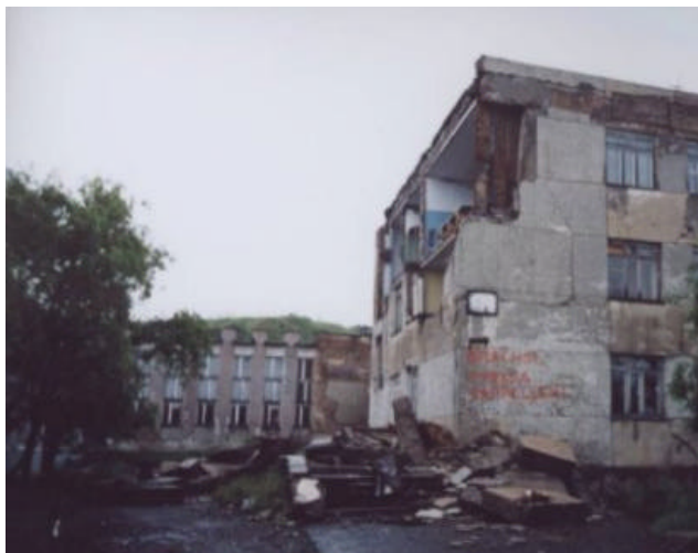
Red paint warns of the potential collapse of these uninhabitable buildings in Tilichiki Settlement of Koryak autonomous region in the Far East of Russian Federation
