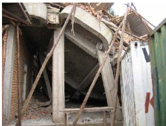
The Sunday, 3 February 2008 earthquake caused extreme and widespread destruction.
