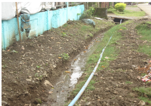
Drainage system that was developed inside the camp (International Federation)
