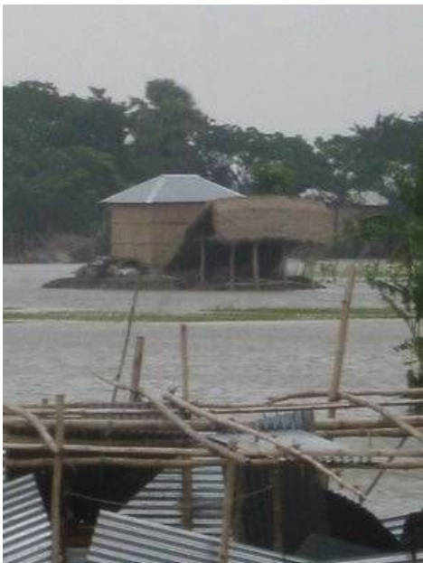
The recently constructed core shelter which, remained intact during Aila. Photo: Bangladesh Red Crescent Society.
