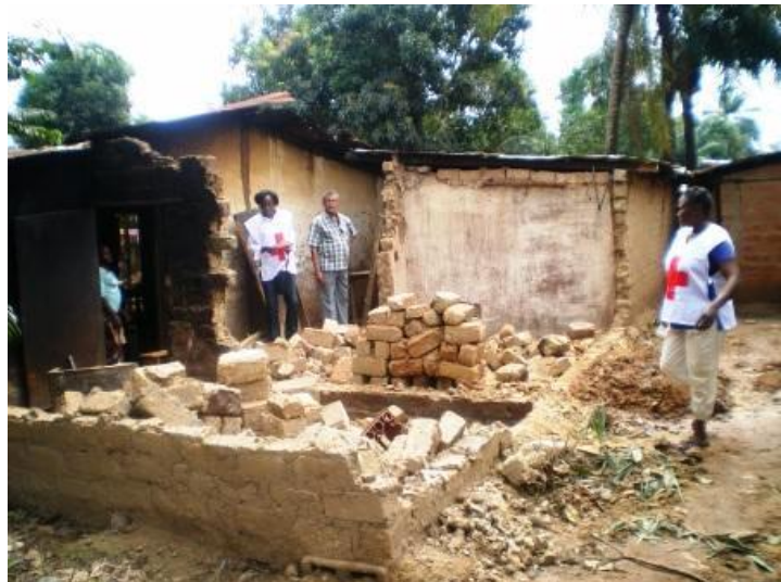
This house, like many others, was destroyed by the storm
