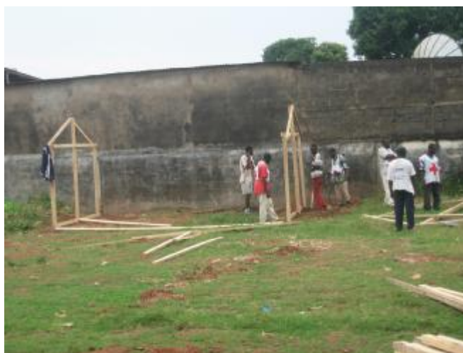
CAR Red Cross volunteers are busy building temporary shelters for the beneficiaries in the site provided by Government Yvette M. Mve/International Federation
