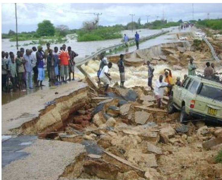
A section of the Malindi - Garsen highway in the coast province that was washed away after heavy rains pounded the area. Photo by KRCS.
