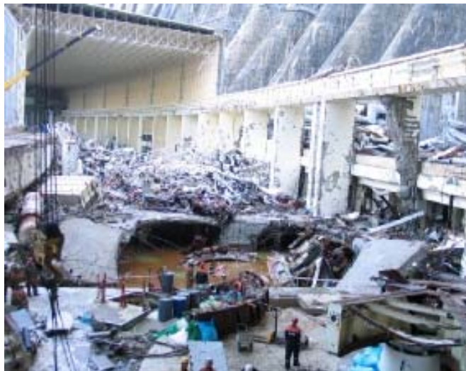
Consequences of the blast in the turbine room at Sayano- Shushenskaya hydropower station. Photo: Russian Ministry of Emergencies
