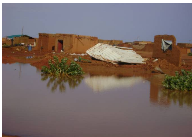
Some of the 21,000 homes damaged from the recent floods.
