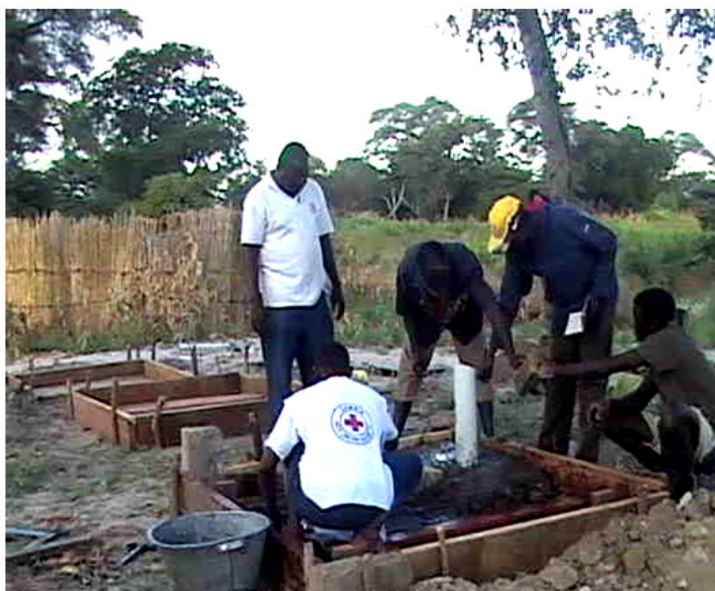
ZRCS staff and volunteers constructing latrines at Mbeta School in Shangombo district in Zambia's Western Province.
