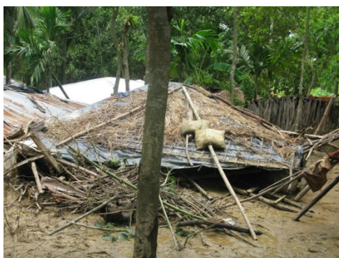
Collapsed house washed away by heavy rain water. Photo: BDRCS/IFRC
