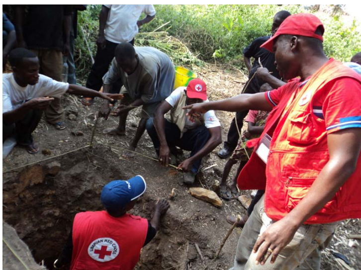
Construction of pit latrines for refugees and host population in Liberia. IFRC/LRCS
