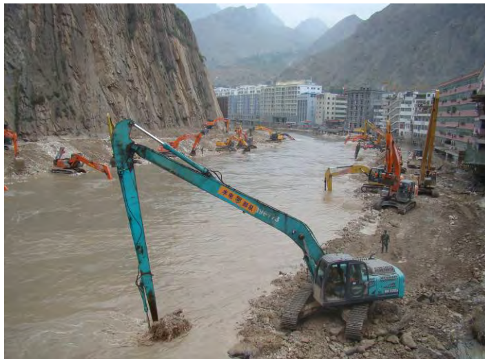
Heavy machineries working alongside Bailong River to clear the barrier lake blocked by tonnes of mud and rocks. Photo: IFRC.
