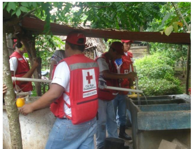
The GRC is performing the cleaning of wells in order to improve the families' quality of life. GRC / F.Cojón
