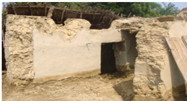
Mud houses cannot withstand gushing water and can be badly damaged. Photo credit: India Red Cross Society
