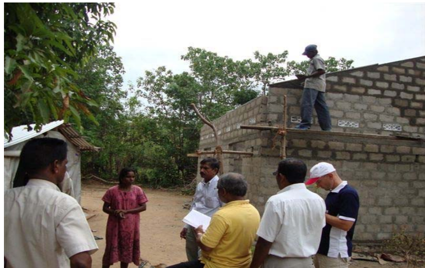
A beneficiary house under construction in Vivekanadanagar. Photo: Sri Lanka Red Cross Society.
