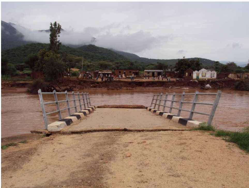
Destroyed Gulwe Bridge which connected Mpwapwa Town with 12 other district wards.
