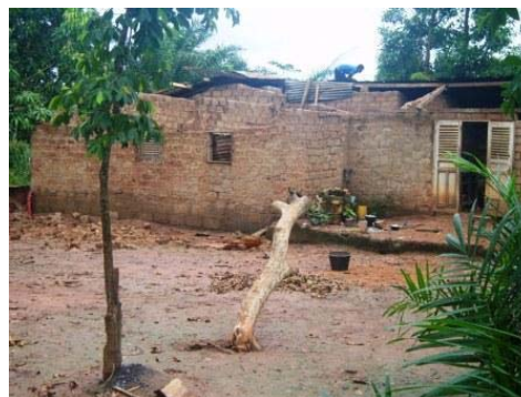
The roof of this house, like many others in Bangui, has been taken away by violent winds / CAR Red Cross
