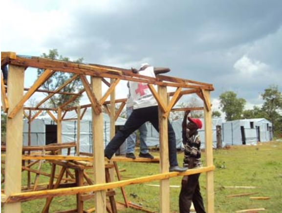
The Red Cross volunteers constructed emergency classrooms to facilitate the return of children to school in Gijia community in Ladduga/NRCS
