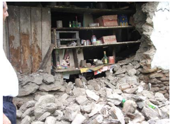
A stone-mud-mortar made house damaged in Dhankuta. Photo: Nepal Red Cross Society.
