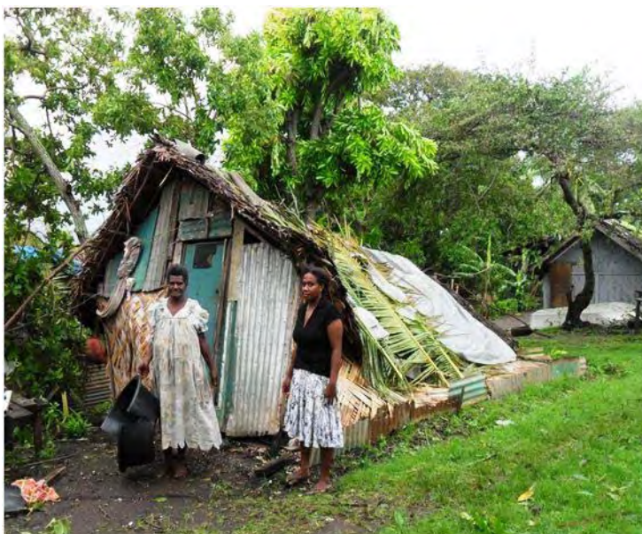
Traditional housing built mainly from thatch, bamboo and grass in Vanuatu has taken a severe beating from the tropical cyclones that have struck the country in the short space of two weeks. (Photo: Vanuatu Red Cross Society)
