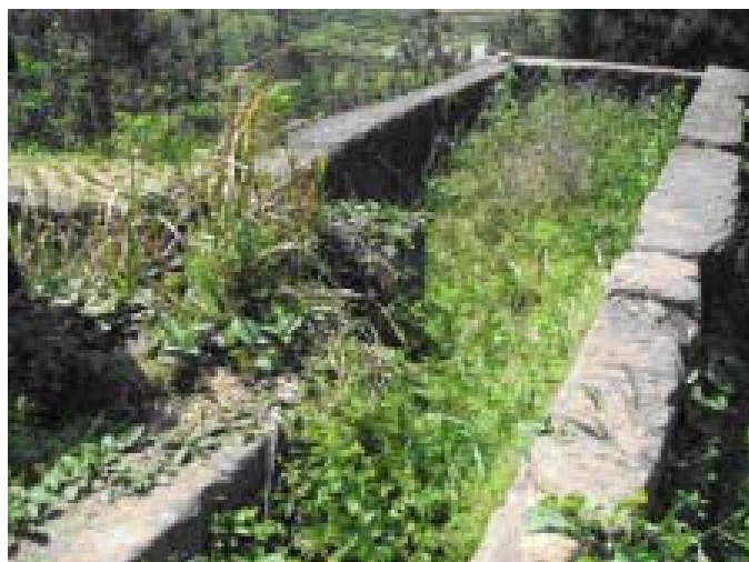
The International Federation's support to the RCSC's community-based disaster preparedness projects will enable Huangjing village in Chongqing to fix and upgrade their water irrigation facilities. April 2008. International Federation.
