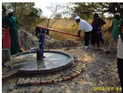
One of the water points constructed in Chikomba district of Mashonaland Central province. A ZRCS volunteer demonstrates how to pump water from the borehole.
