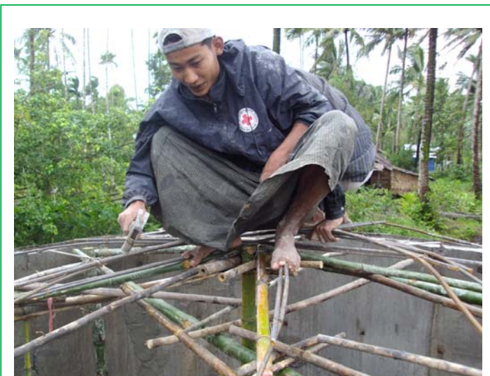
A volunteer hard at work during the construction of a water tank in Kapanan village in Bogale township, in July this year: Trained volunteers are part of water and sanitation teams in all nine hubs in Nargis-affected areas. The teams represent the elevated capacity of the Myanmar Red Cross Society in the water, sanitation and hygiene promotion sector. (Photo: Si Thu Tun/Myanmar Red Cross Society)
