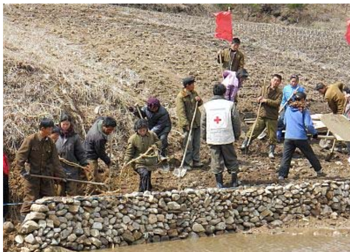
Construction of a riverbank reinforcement, to mitigate the impact of possible flooding in Chusang ri, Hamju county, South Hamgyong province Photo: Won Jong Chol, DPRK Red Cross/South Hamgyong branch
