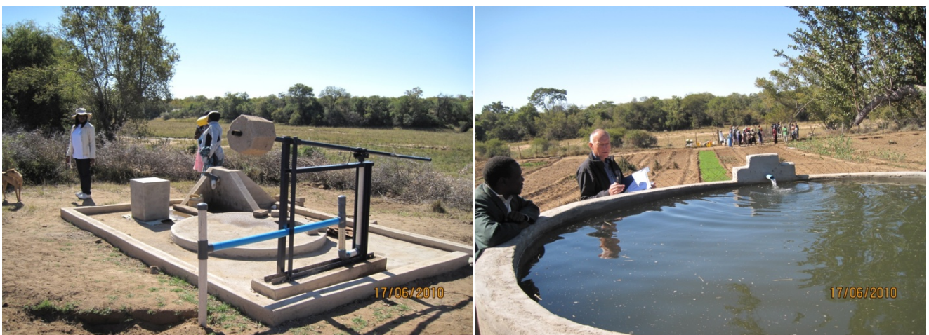
Sand Water Abstraction pump and tank in Rural Gwanda, Matabeleland South
