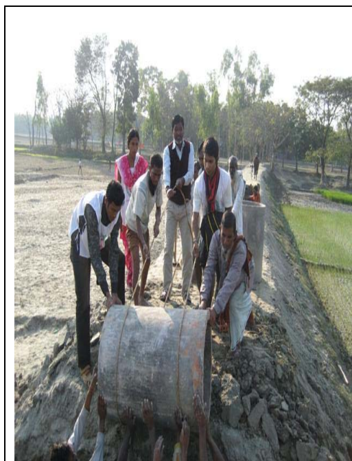
Community people and volunteers constructing a new earthen road under the climate change adaptation programme. Photo: IFRC.
