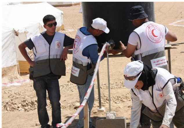
PRCS volunteers practicing in water and sanitation as part of the training to become National Disaster Response Teams (NDRT) in Bein Na'im, near Hebron – photo: PRCS, June 2011
