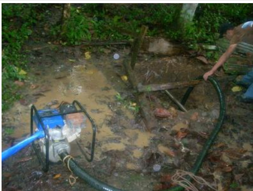
Costa Rican Red Cross volunteers cleaning mud out of a water well in the Upala community. Source: CRRC
