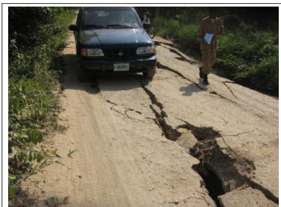
A damaged road in Puerto Cortes. Source: Honduran Red Cross
