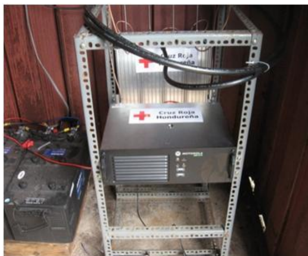
Repeater installed in the Cerro Negro mountain in the department of Copan. Source: Honduran Red Cross
