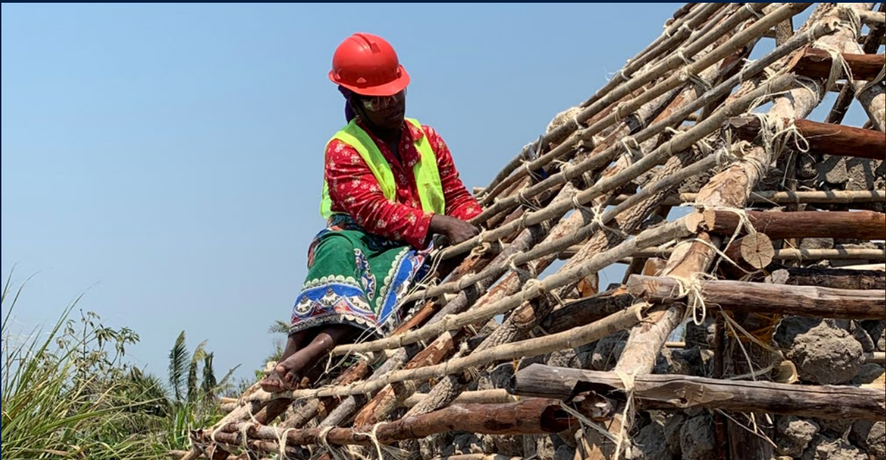
Mozambique 2019 A skilled worker tying joists. At the beginning of the project female workers were afraid to work on the roof, but as their skills improved they became comfortable to climb to the top of the structure. © Jenn Houtby / IFRC
